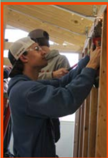
Reese Gingerich adds hurricane clips to the roof of the seed shed in construction class. Photo by Olivia Naber.
